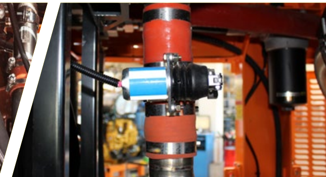
Air shutoff valve
