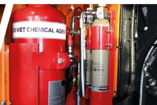
Automatic fire-extinguishing system
